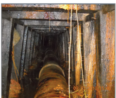
Original, deteriorating tunnel
